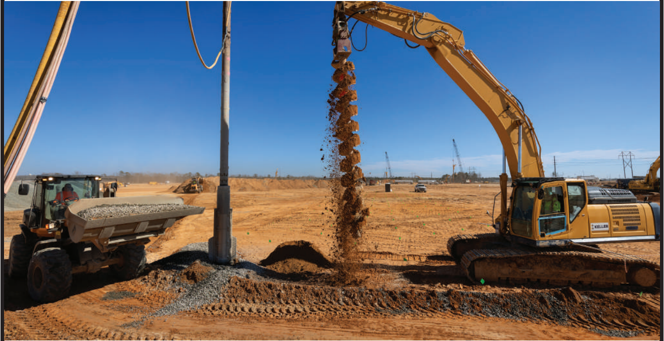
Keller North America ( No. 17 ) is providing ground improvement services over approximately 15 million sq ft of building pads on the $2-billion Scout Motors electric vehicle plant in Blythewood, S.C. The primary scope of work is the installation of aggregate piers with varying depths of 5-30 ft. The facility is scheduled to start production in 2026.
