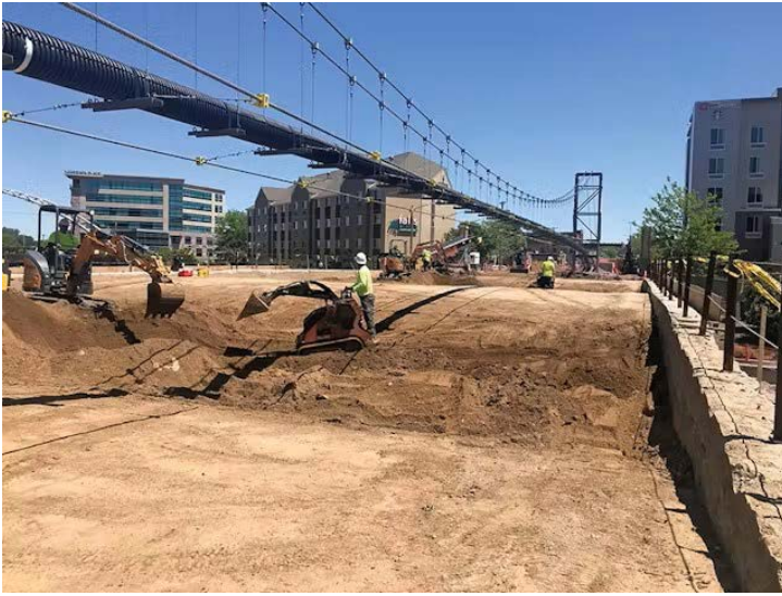
Temporary Cable Suspension System
