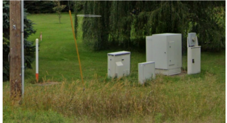
Digital Loop Carrier System DSL Electronics Cabinet
