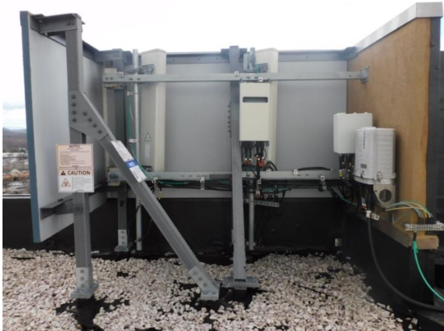
Figure 3. Image of a typical rooftop FRP concealment frame
