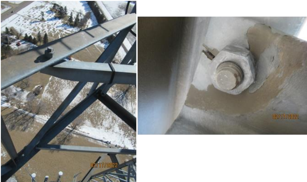
Figure 20. Images of cracked standoff member and plastic deformation.
