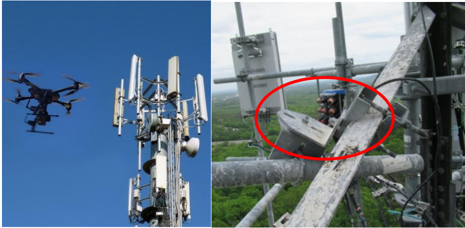
Figure 31. Image of drone inspecting a tower and a structural fault
