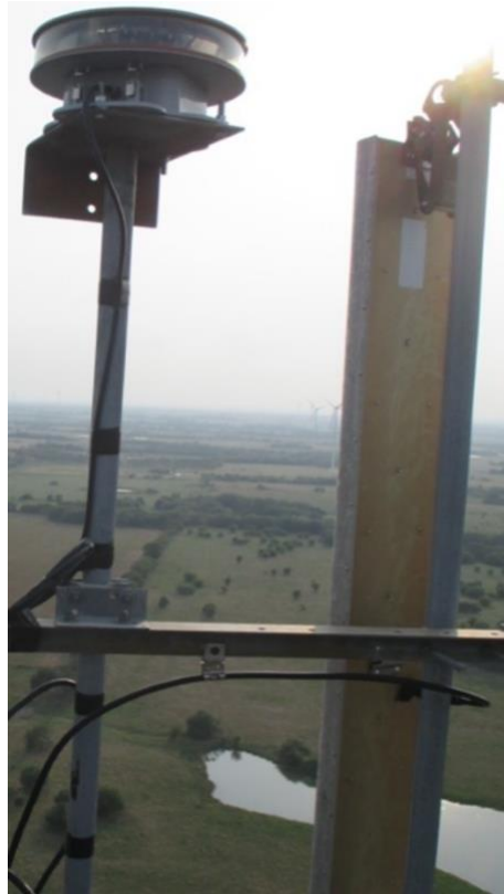
Figure 12. Image of mount components and/or equipment placement violates FAA requirements
