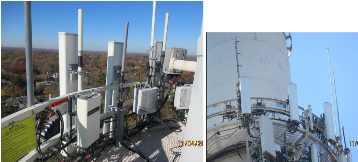
Figure 17. Images of a round platform with equipment installed at the ~223 ft elevation on the smokestack structure shared by two MNOs.
